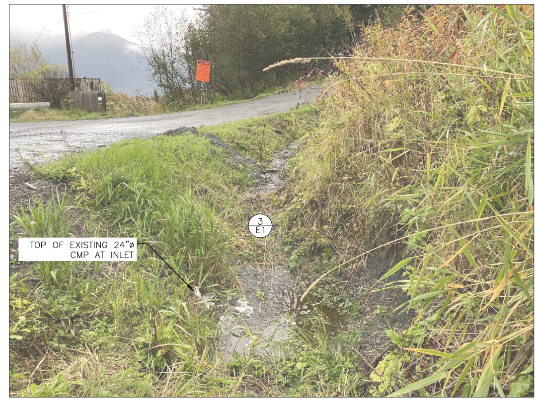
3 F1 BEACH ROAD CULVERT REPLACEMENT, EXISTING DITCH LOOKING UPHILL SCALE: N.T.S., LATITUDE: 59.224262°, LONGITUDE: -135.416568°
